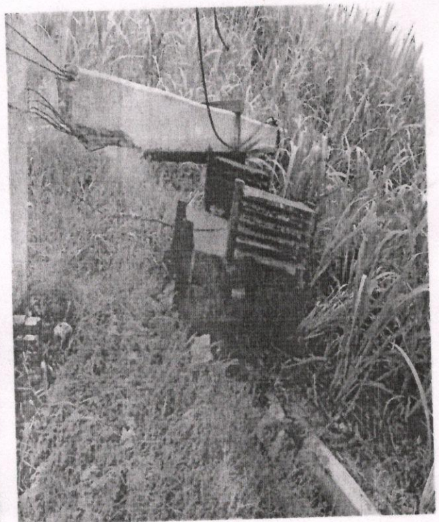
Figure 08 damaged electric pole
