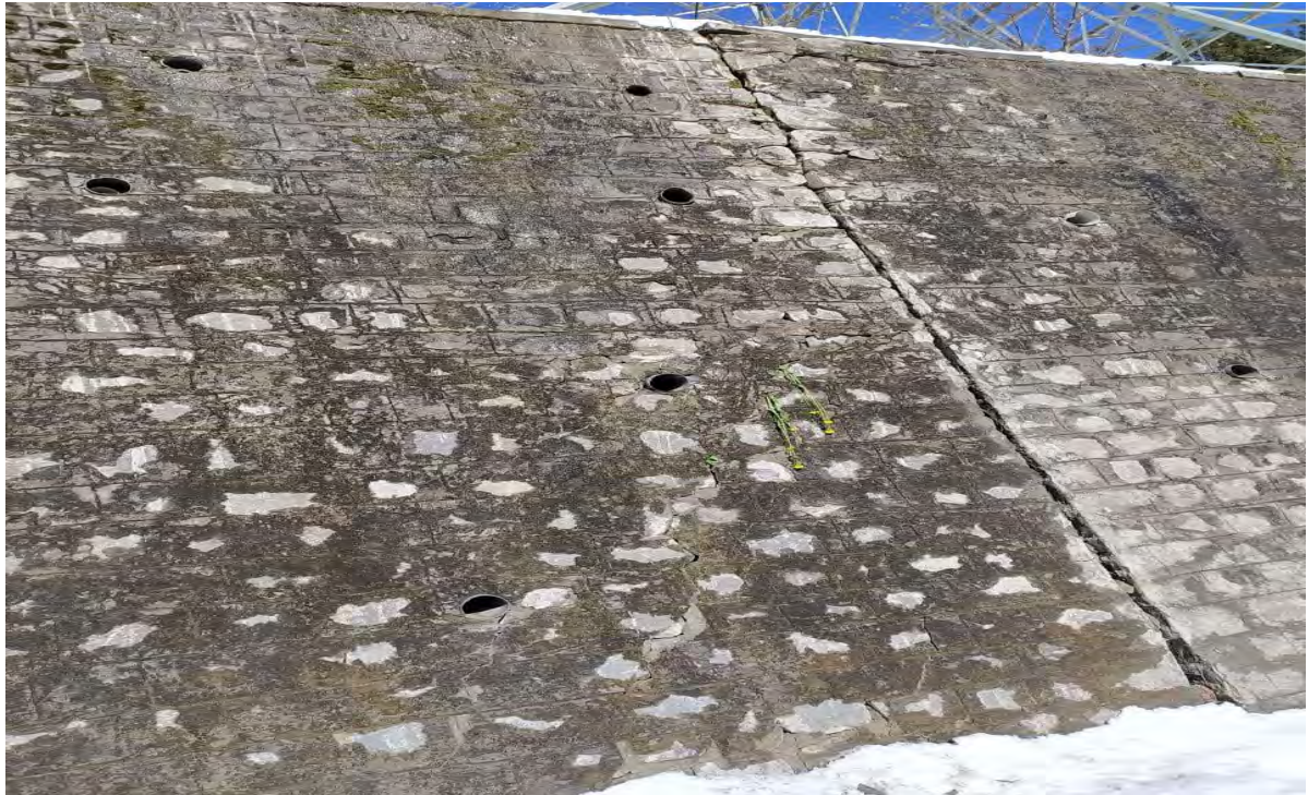
Fig:- Photograph showing cracks
