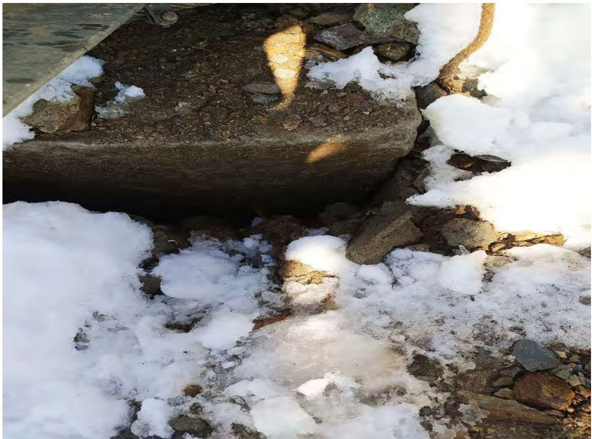
Fig:- Photograph showing settlement of soil.
