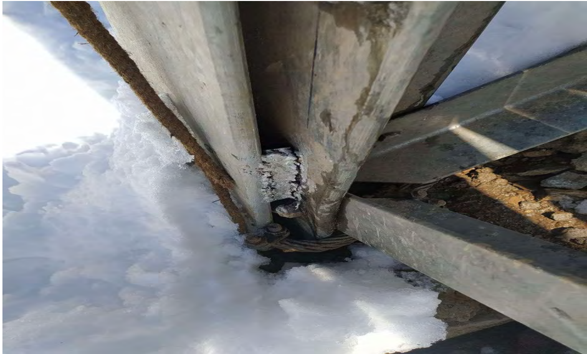
Fig:- Photograph showing stress in welded joints.
