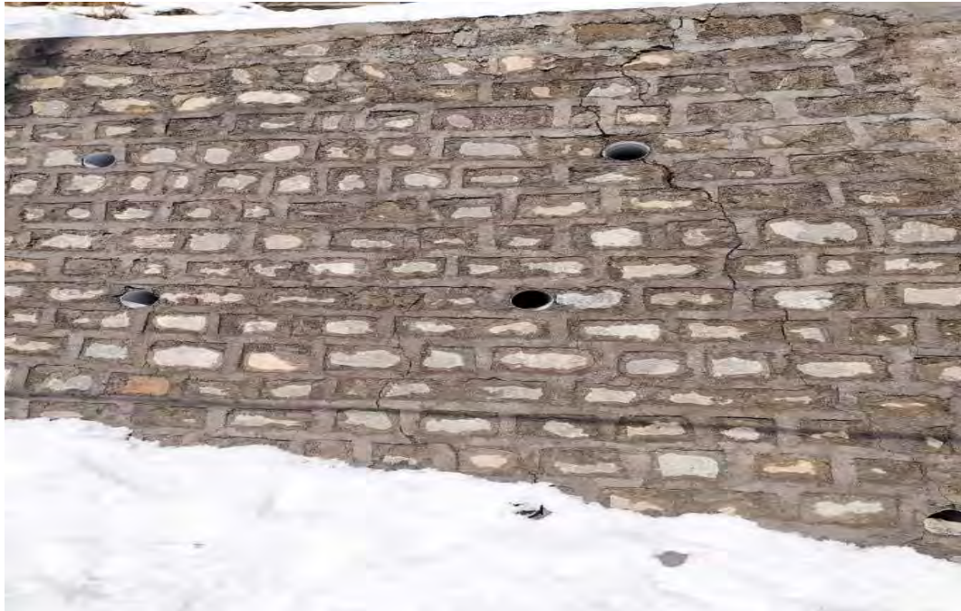
Fig: - Photograph showing cracks in new revetment.
