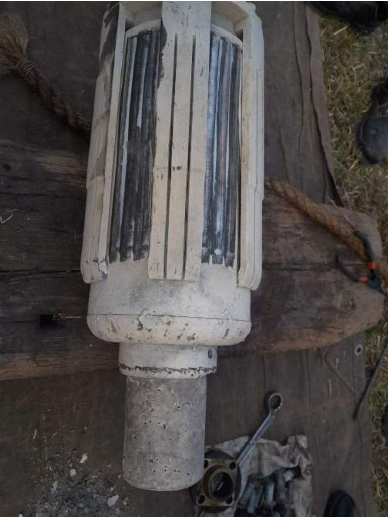
220kV Kharar Bay R-phase Breaker
