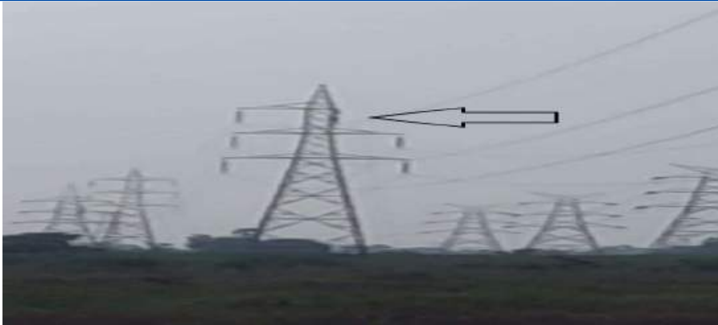
Damaged cross arm
