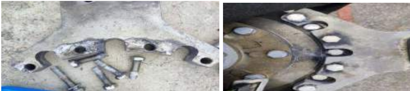
Damaged trip coils and breaker pad
